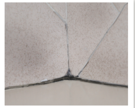
Black Mold Caulking at Tub Deck
